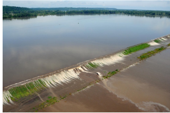
Photo 18. Levee overtopping. Source: USACE
